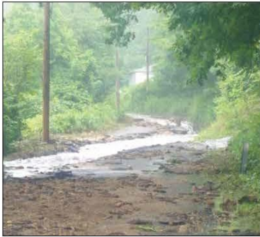
Water coming down Coy Hill cut through O'Neil Road, removing the road surface. Photo Courtesy of James McKeon
